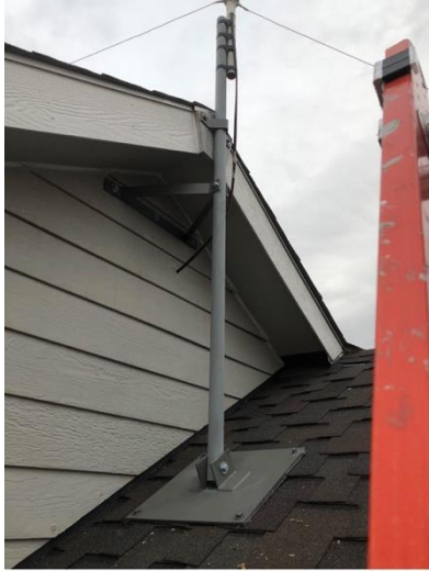
Figure 1. The custom roof mounting system.
