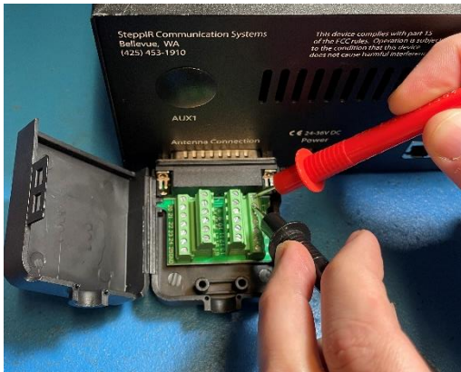
Figure 5: Spare DB25 field splice voltage measurements
